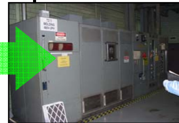
2000A 3Ø Switchgear
