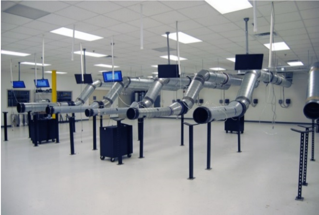
Venturi Calibration Room
